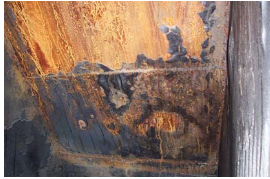
Photo 2: Flue gas moisture condensation inside duct
