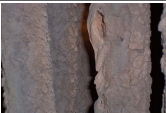
Photo 11: Ash builds up on convective Surface – inadequate furnace volume
