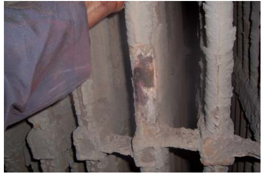
Photo 8: Fouling & corrosion over superheater
