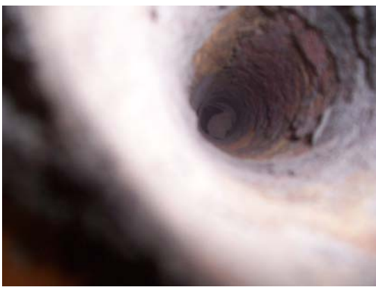
Photo 3: Ash build up due to moisture condensation inside APH tubes
