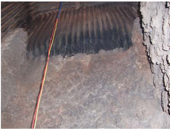
Photo 9: Furnace ash slagging since the waterwall surface is inadequate.
