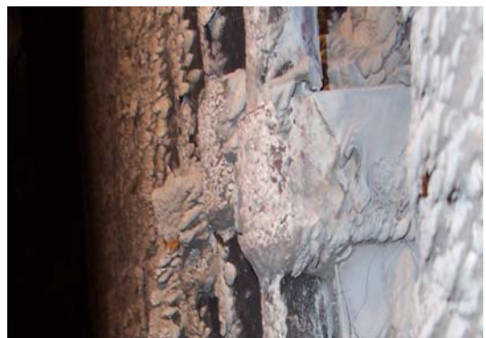
Photo 6: Ash build up over superheater due to inadequate furnace volume / water wall.
