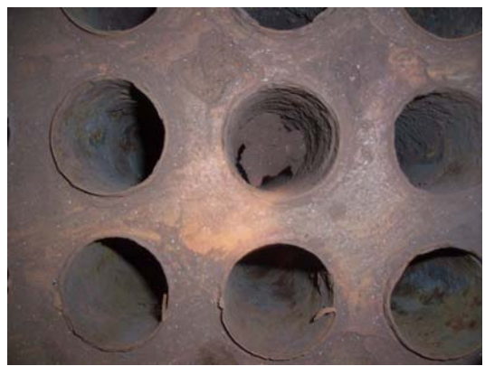
Photo 4: APH metal loss due to moisture condensation
