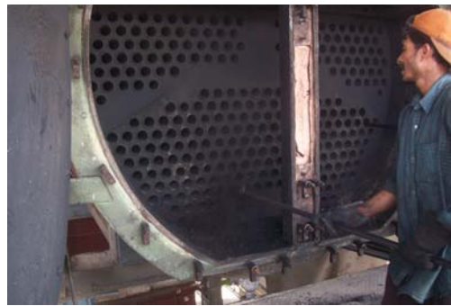
Photo 10: frequent shell tube cleaning calls for disturbance in plant.
