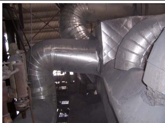
Photo 18: Air ingress from roof in a boiler designed for paper mill.
