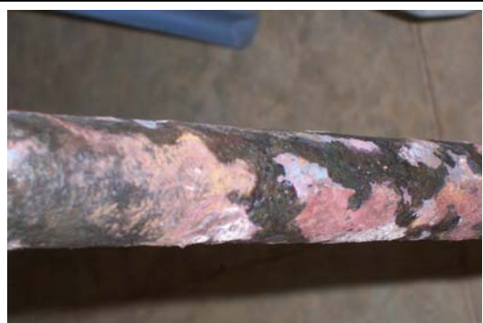
Photo 12: Superheater tube corrosion due to alkaline chloride corrosion.
